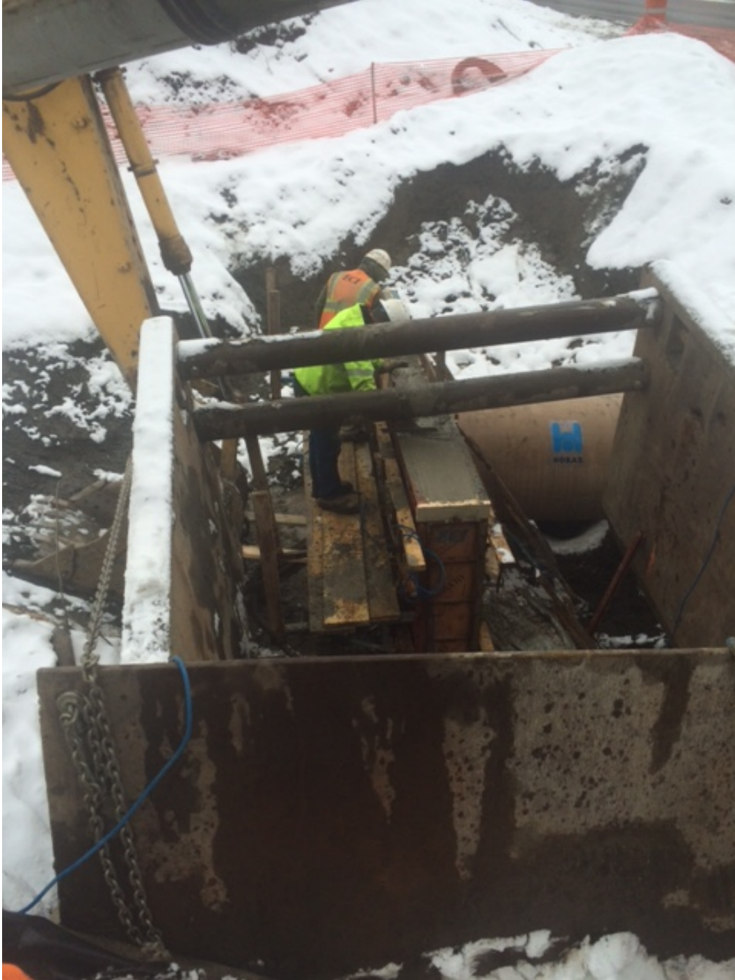
"Construction workers are finishing the top surface of the headwall (center of photo) to 42" drainage pipe."
